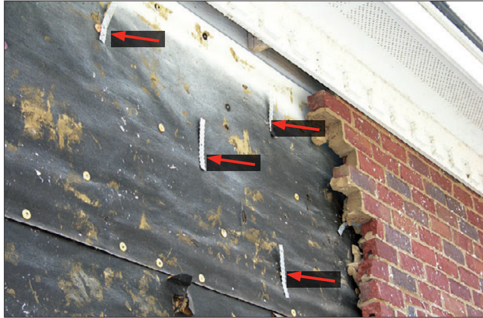
Figure 6-58: The four ties shown by the red arrows were not embedded into the mortar. Estimated wind speed: 105 mph. Hurricane Katrina, (Mississippi, 2005)
