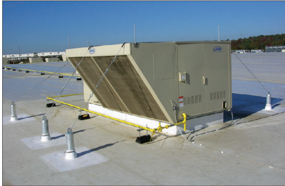
Figure 6-135: To strengthen attachment of this HVAC unit, robust pipe anchors were attached to the deck and cables with turnbuckles installed.
