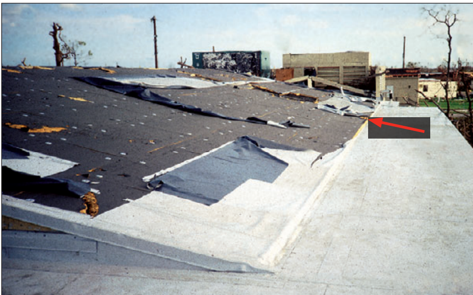
Figure 6-85: This mechanically attached single-ply membrane progressively tore after being cut by wind-borne debris. Hurricane Andrew (Florida, 1992)
