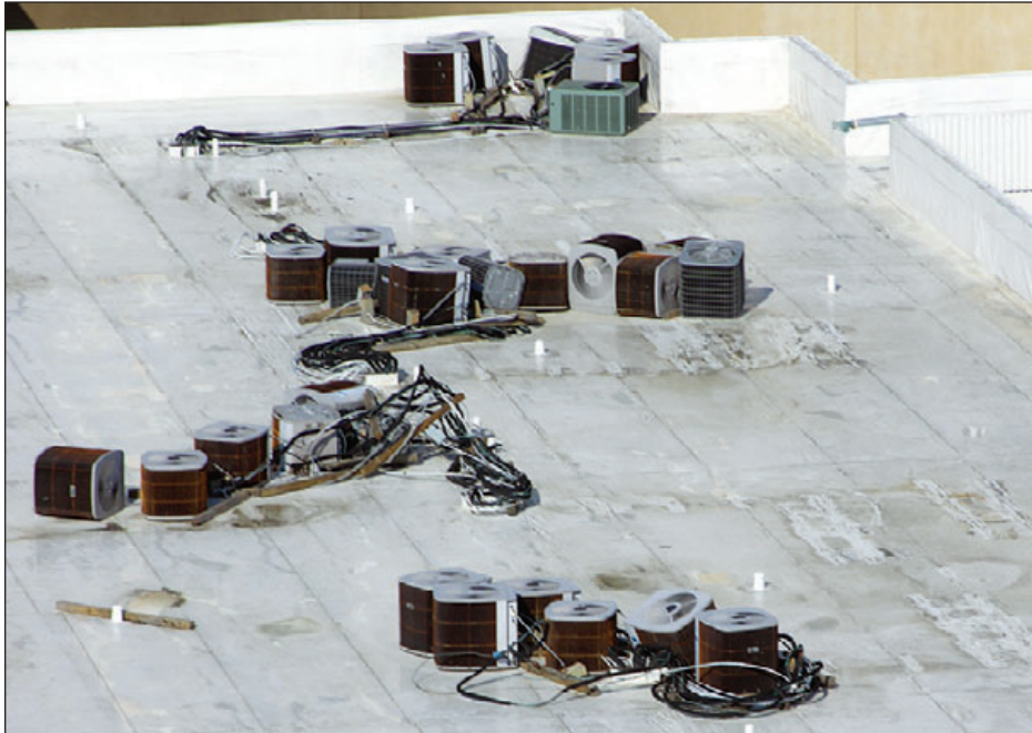
Figure 6-94: These condensers were blown off their sleepers. Displaced condensers can rupture roof membranes and refrigerant lines. Estimated wind speed: 120 mph. Hurricane Katrina (Mississippi)
