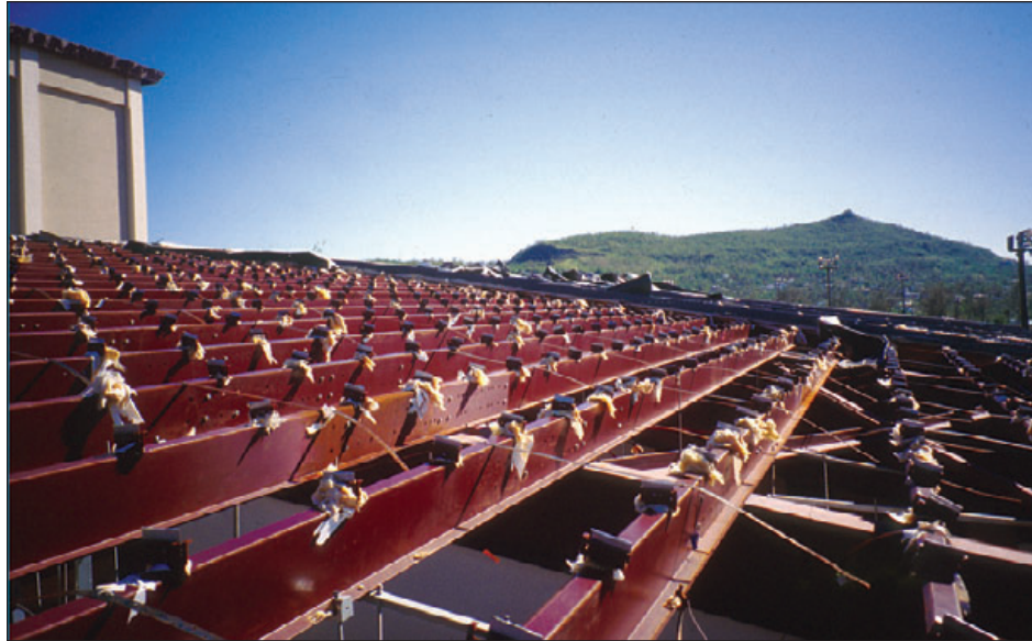
Figure 6-20: This newly-constructed gymnasium had a structural metal roof panel (3-inch trapezoidal ribs at 24 inches on center) applied over metal purlins. The panels detached from their concealed clips. A massive quantity of water entered the school and buckled the wood gym floor. Typhoon Paka (Guam, 1997)
