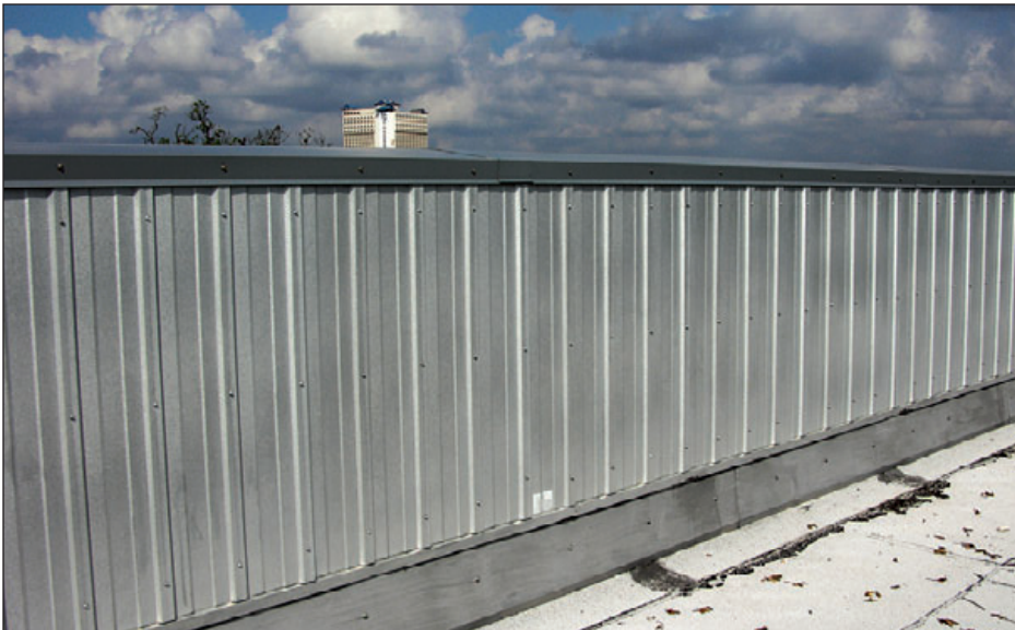
Figure 6-88: Base flashing protected by metal wall panels attached with exposed screws. Estimated wind speed: 120 mph. Hurricane Katrina (Mississippi, 2005)
