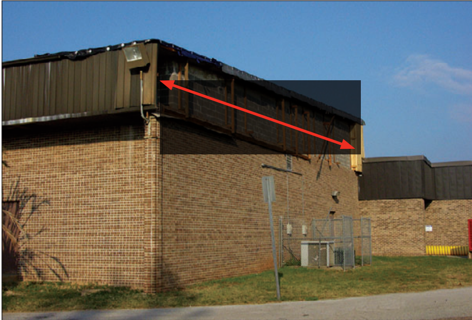
Figure 6-65: Blow-off of metal fascia panels due to inadequate attachment of wood furring to the CMU wall. Estimated wind speed: 85–95 mph. Hurricane Ivan (Florida, 2004)
