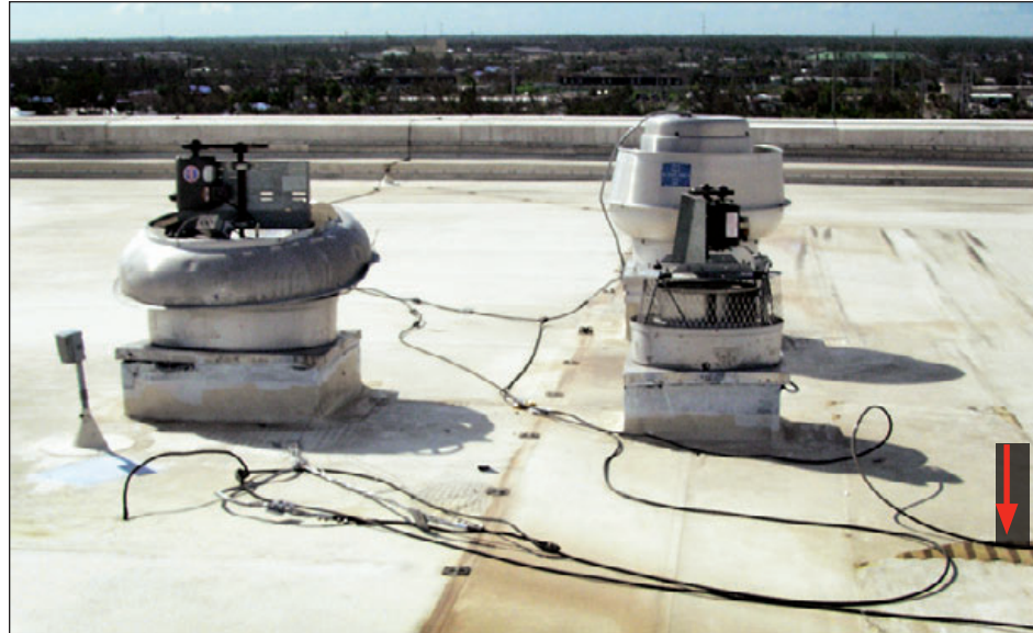
Figure 6-92: Cowlings blew off two of the three fans. Note also the loose LPS conductors and missing walkway pad (red arrow). Estimated wind speed: 140–160 mph. Hurricane Charley (Florida, 2004)
