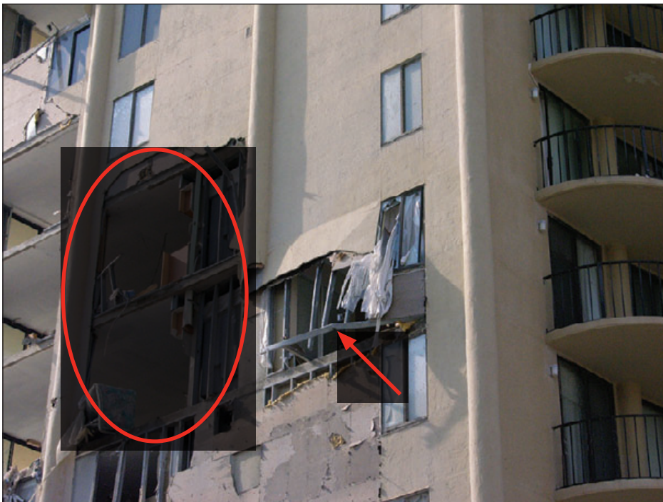
Figure 6-63: The stucco wall failure was caused by inadequate attachment between the stud tracks and the building's structure. All of the metal stud framing within the red oval blew away. The arrow shows a bottom stud track that detached and pulled away from the building. Estimated wind speed: 110–125 mph. Hurricane Ivan (Florida, 2004)
