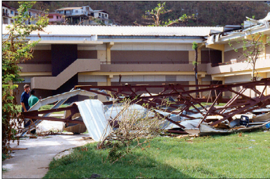
Figure 6-122: The steel truss superstructure installed on this school as part of a steep-slope conversion blew away because of inadequate attachment. Hurricane Marilyn (U.S. Virgin Islands, 1995)
