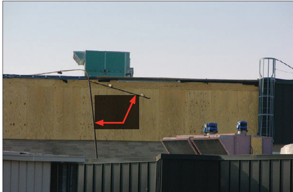
Figure 6-99: The school shown in Figures 6-65 and 6-98 also experienced gas line rupture (shown by the lines dangling over the side of the building). Estimated wind speed: 85–95 mph. Hurricane Ivan (Florida, 2004)
