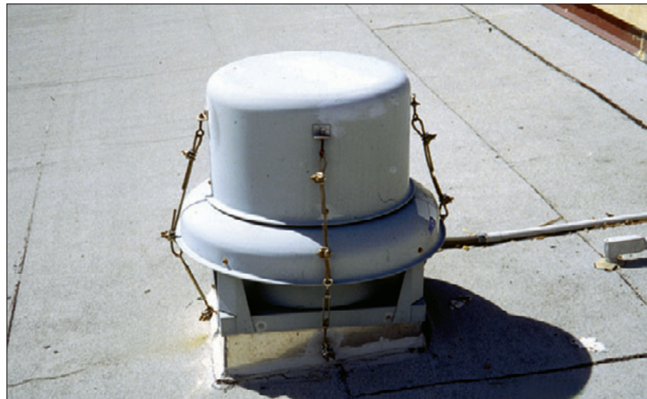
Figure 6-93: Cables were attached to prevent the cawling from blowing off. Typhoon Paka (Guam, 1997)
