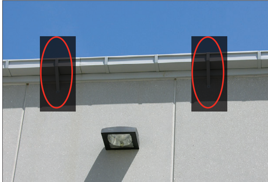
Figure 6-77: Sheet metal straps were attached to an existing gutter that lacked sufficient uplift resistance.
