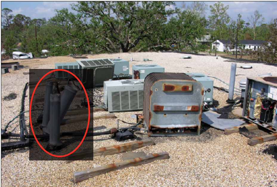
Figure 6-137: These condensers were simply mounted on wood sleepers that rested on the roof surface. Note the damaged exhaust stacks and missing rain caps (red oval). Estimated wind speed: 105 mph. Hurricane Katrina (Mississippi, 2005)
