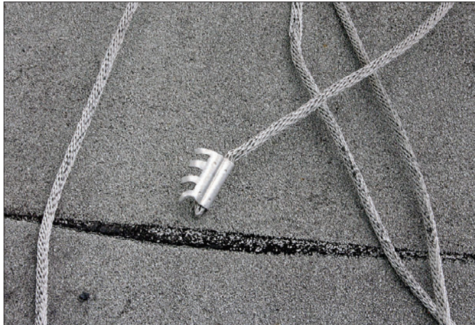
Figure 6-116: If conductors detach from the roof, they are likely to pull out from pronged splice connectors. Estimated wind speed: 90–100 mph. Hurricane Charley (Florida, 2004)
