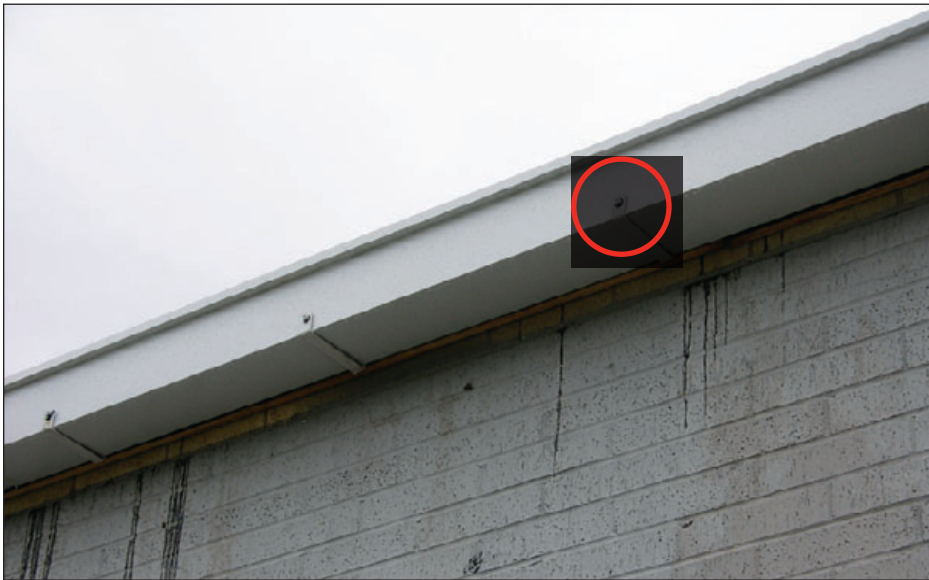
Figure 6-76: At this gutter, a fastener connected the bracket to the gutter. Note: To avoid leakage at the fasteners between the bracket and gutter, the bracket should extend near or to the top of the gutter so that the fastener would be above the waterline. Estimated wind speed: 95 mph. Hurricane Ike (Texas, 2008)
