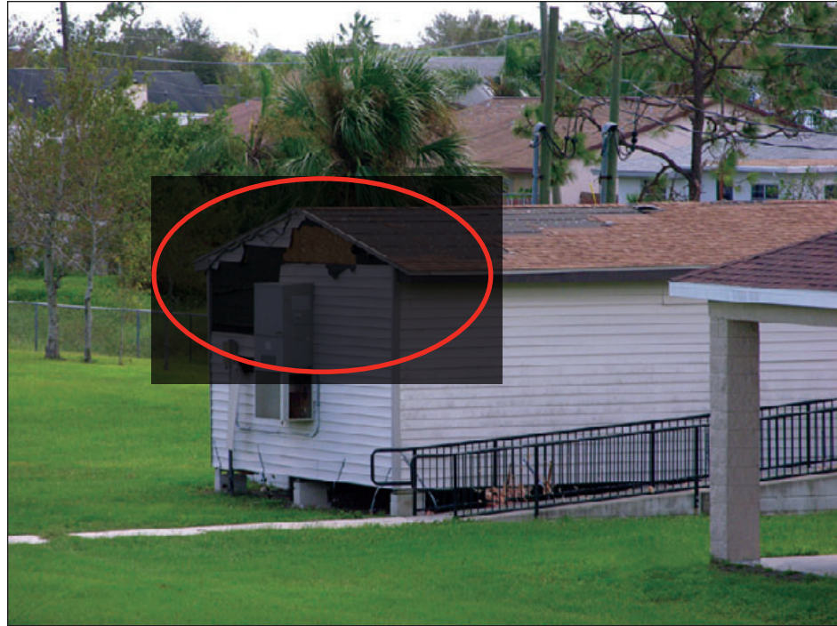
Figure 6-28: Asphalt shingles and vinyl siding blew off of this portable classroom. This type of wind-borne debris can break unprotected glazing. Hurricane Francis (Florida, 2004)
