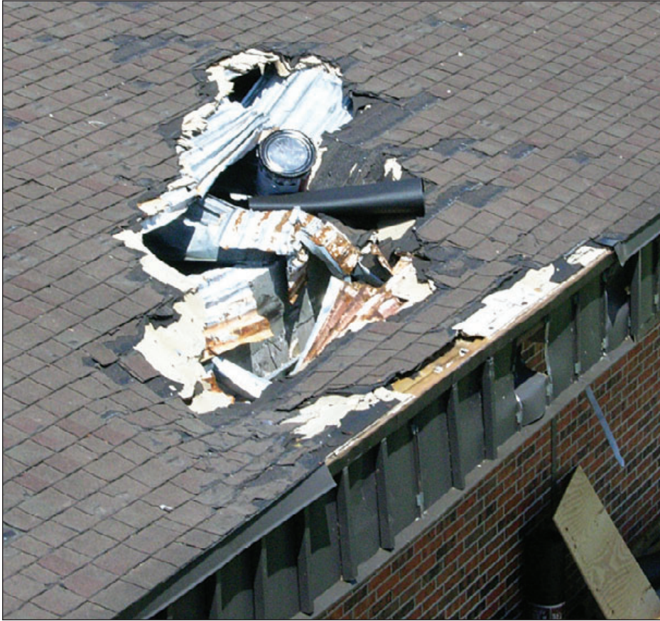
Figure 6-42: At the school shown in Figure 6-34, wind-borne debris ruptured the proprietary composite deck system composed of light gauge corrugated metal deck and gypsum board. Estimated wind speed: 140 to 160 mph. Hurricane Charley (Florida, 2004)
