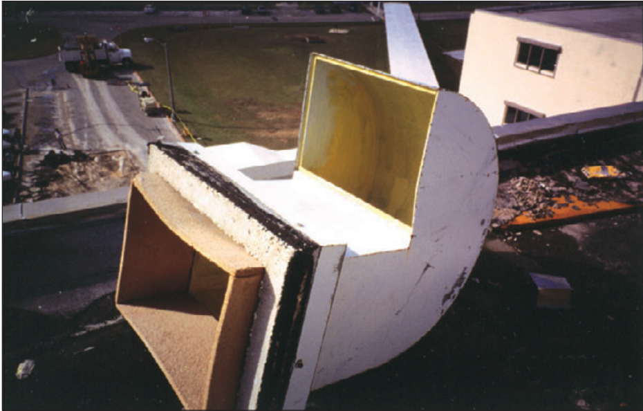
Figure 6-91: The gooseneck on this building remained attached to the curb, but the curb detached from the deck. Typhoon Paka (Guam, 1997)
