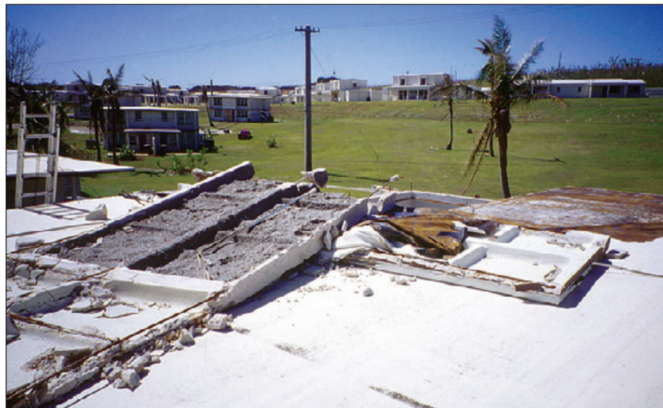
Figure 6-39: Portions of this waffled precast concrete roof deck were blown off. Typhoon Paka (Guam, 1997)
