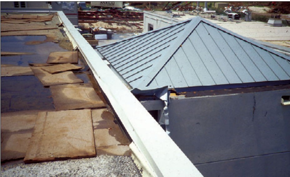
Figure 6-9: The irregularity created by the stair tower (covered with a metal roof) caused turbulence resulting in wind speed-up and roof damage. Hurricane Andrew (Florida, 1992)
