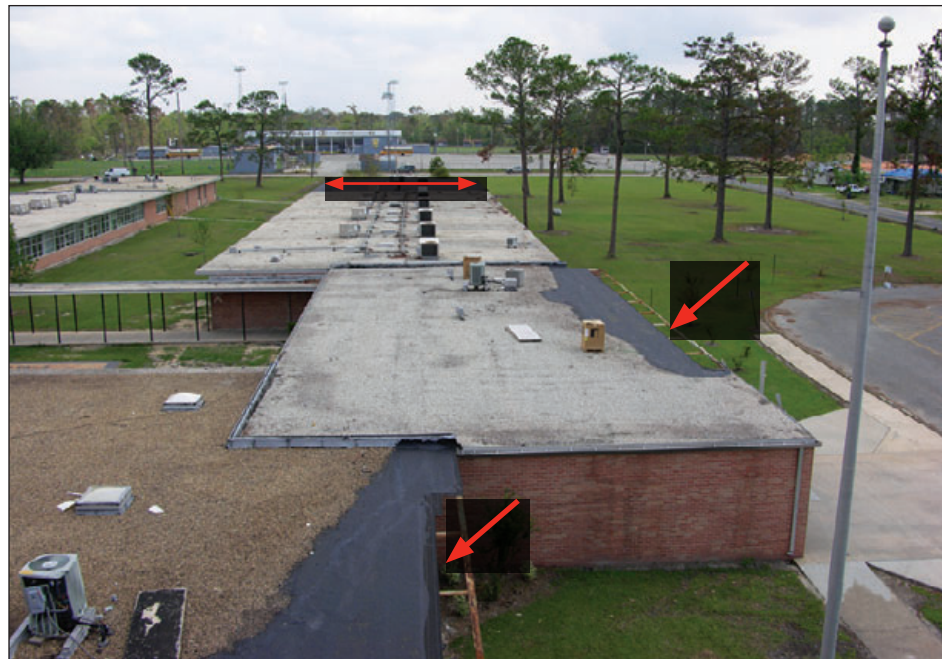
Figure 6-26: The cementitious wood-fiber deck panels blew off the overhangs and caused a progressive lifting and peeling of the roof membrane. Strengthening (or replacing) inadequately attached roof decks during a reroofing project is both prudent and relatively economical. Estimated wind speed: 120 mph. Hurricane Katrina (Mississippi, 2005)
