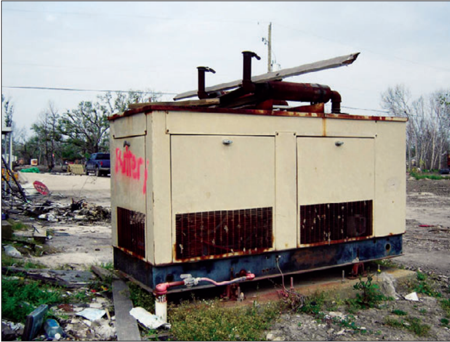
Figure 5-19: Although it was anchored and not displaced by floodwaters, this generator was out of service after being submerged (Hurricane Katrina, 2005)
