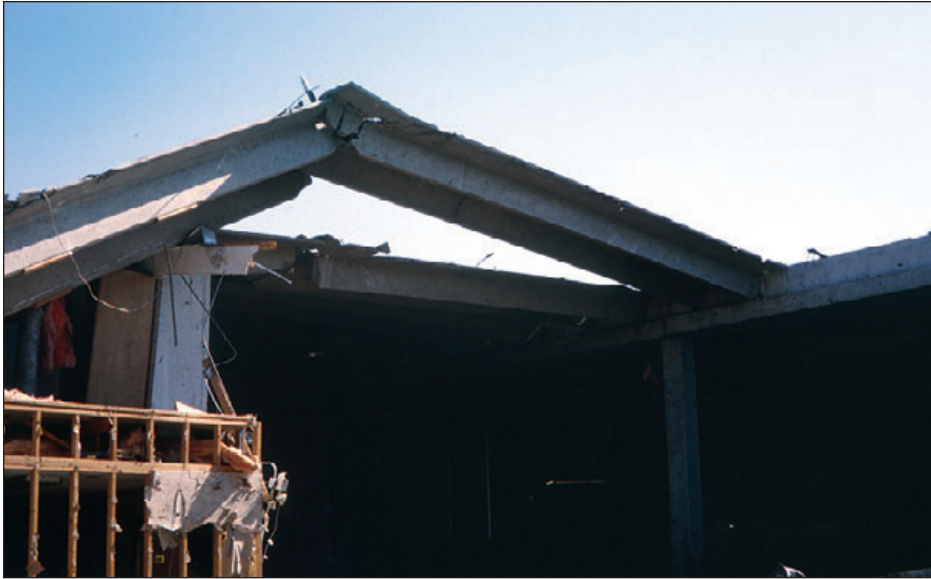
Figure 6-40: Twin-Tee roof panel lifted as a result of the combined effects of wind uplift and pre-tension. Tornado (Missouri, May 2003)
