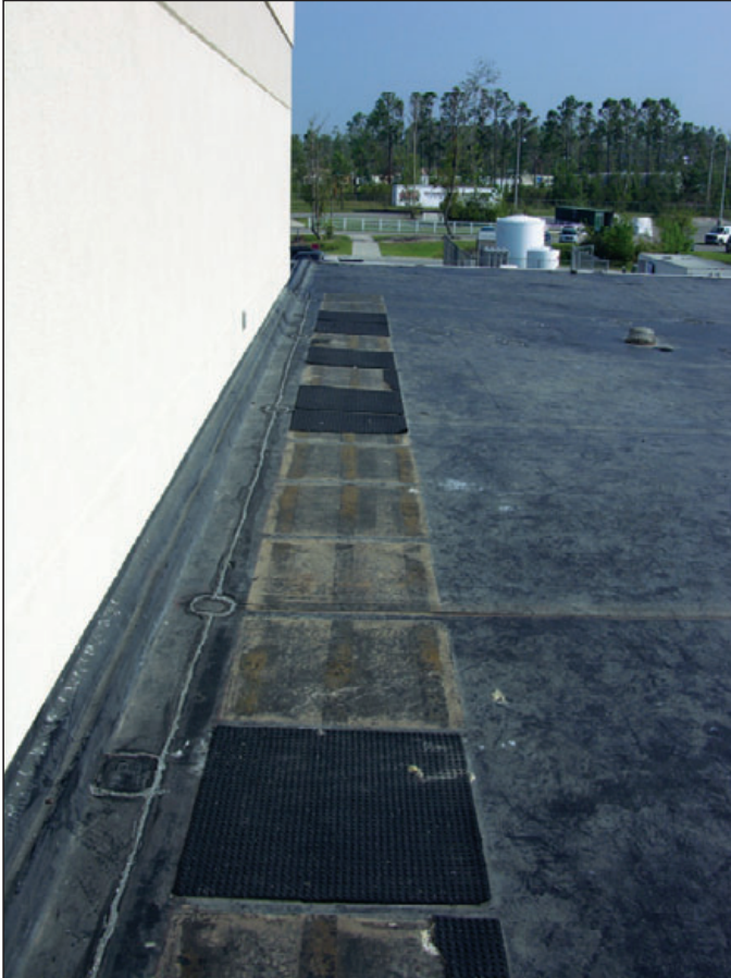
Figure 6-87: Several rubber walkway pads were blown off the single-ply membrane roof. Estimated wind speed: 130 mph. Hurricane Katrina (Mississippi, 2005)
