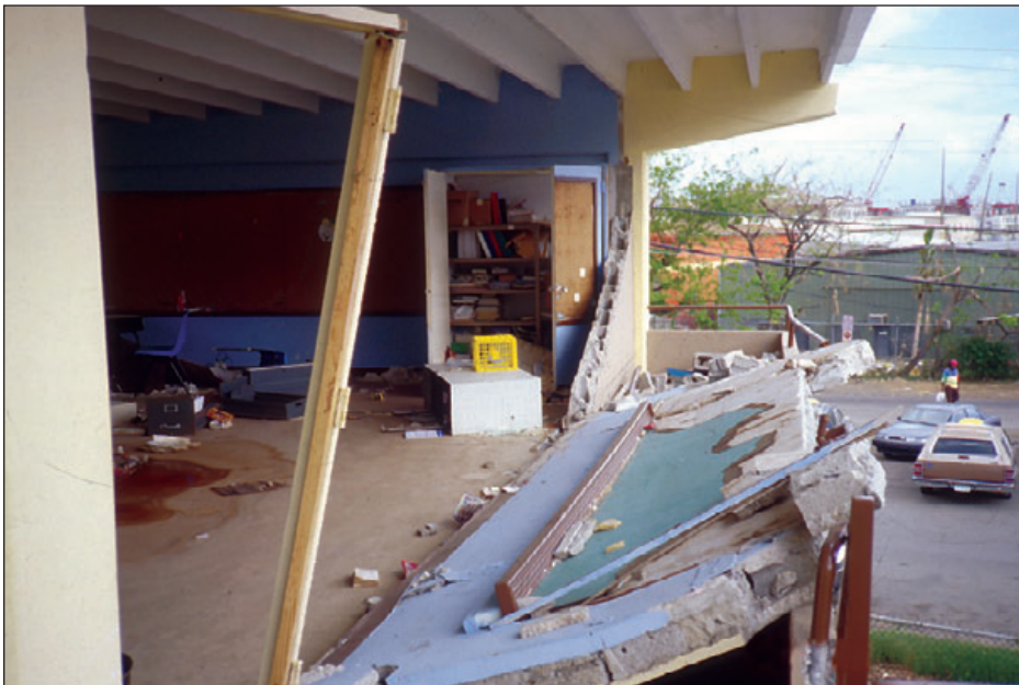
Figure 6-16: Collapsed unreinforced CMU wall. Hurricane Marilyn (U.S. Virgin Islands, 1995)
