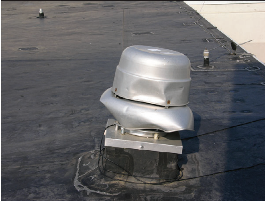
Figure 6-103: This exhaust fan was impacted by wind-borne debris. Although it is often impractical to place all equipment such as fans in penthouses, doing so to the extent possible avoids debris damage. Estimated wind speed: 130 mph. Hurricane Katrina (Mississippi, 2005)
