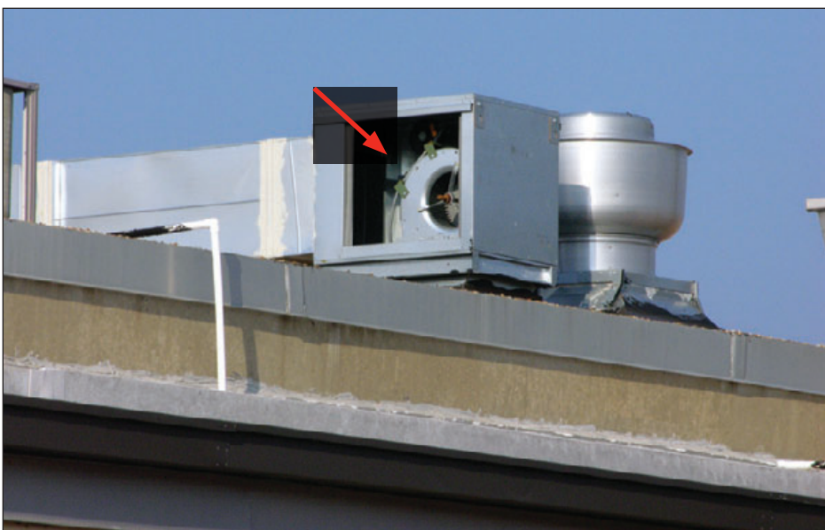
Figure 6-98: The school shown in Figure 6-65 also had an access panel blow off. Blown-off panels can puncture roof membranes, break glazing, and cause injury. Estimated wind speed: 85–95 mph. Hurricane Ivan (Florida, 2004)
