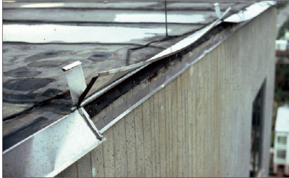
Figure 6-71: The metal edge flashing on this building disengaged from the continuous cleat and the vertical flange lifted. Hurricane Hugo (South Carolina, 1989)
