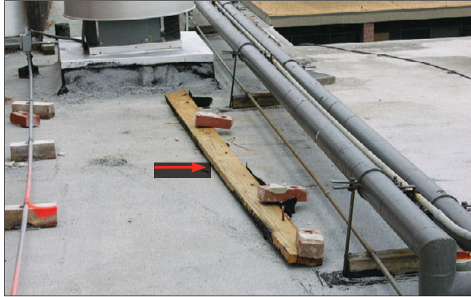
Figure 6-132: The nailer (red arrow) blew off an upper roof and landed on the roof below. The nailer was anchored to a brick wall. Some of the anchors pulled out of the brick, and some of the bricks blew away with the nailer. Estimated wind speed: 105–115 mph. Hurricane Ivan (Florida), 2004
