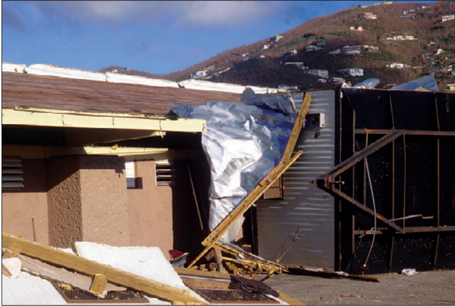
Figure 6-19: This portable classroom was blown up against the main school building. Depending upon the type of exterior wall, an impacting portable classroom may or may not cause wall collapse. Hurricane Marilyn (U.S. Virgin Islands, 1995)
