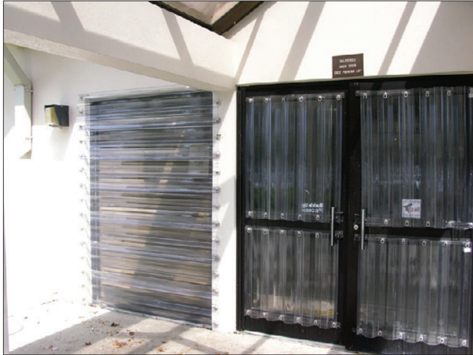
Figure 6-127: Polycarbonate shutters were temporary screwed to the doors and wall adjacent to the window opening. An advantage of polycarbonate is its translucence, which allows daylight to enter the building without removing the shutters. Hurricane Francis (Florida, 2004)
