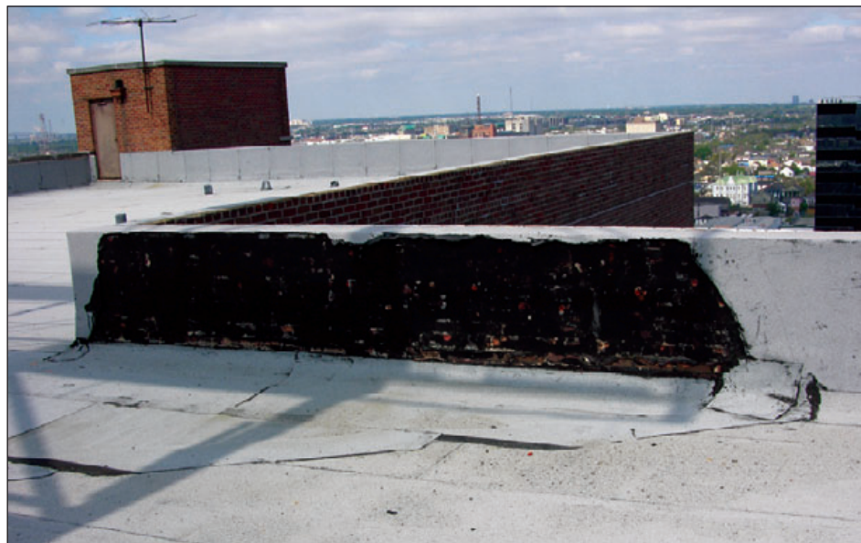
Figure 6-133: Failed base flashing adhered directly to the brick parapet. Estimated wind speed: 105 mph. Hurricane Katrina (Louisiana, 2005)
