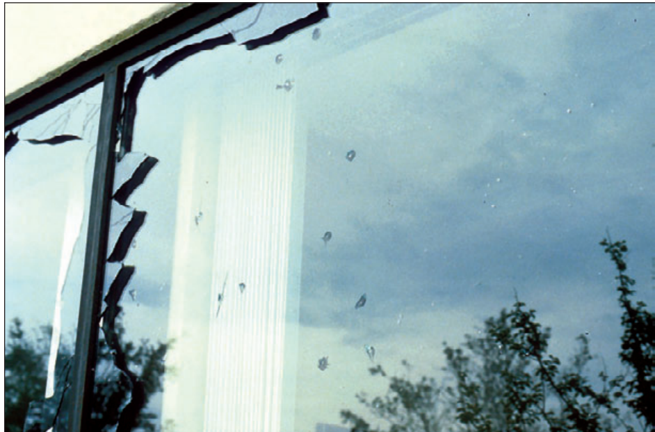
Figure 6-14: The outer window panes were broken by aggregate from a built-up roof. Estimated wind speed: 104 mph. Hurricane Hugo (South Carolina, 1989)
