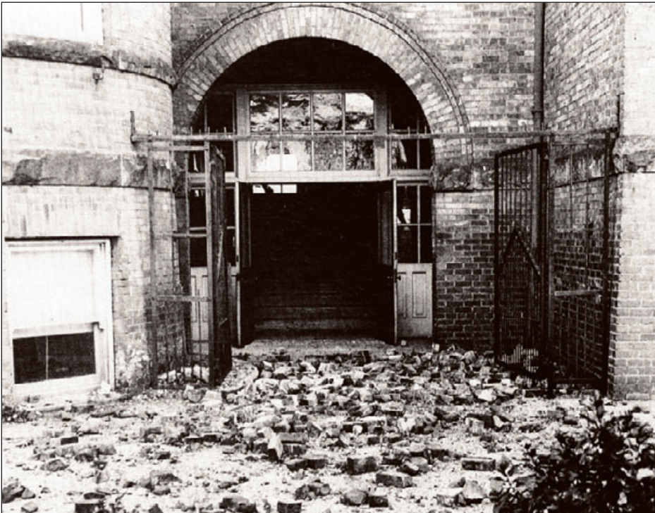
Figure 4-20: Another dangerous entry collapse, Seattle, WA, 1949
