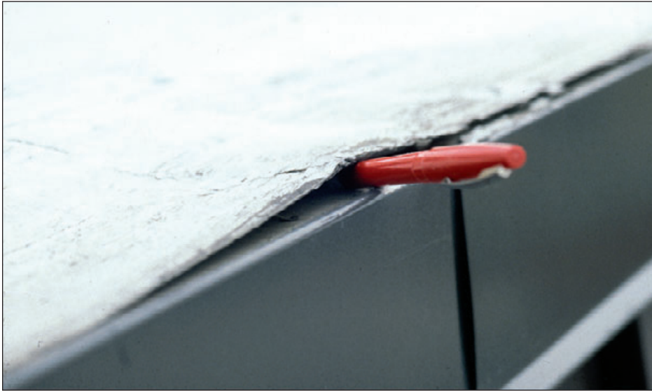
Figure 6-70: The ink pen shows an opening that the wind can catch to cause lifting and peeling of the membrane.
