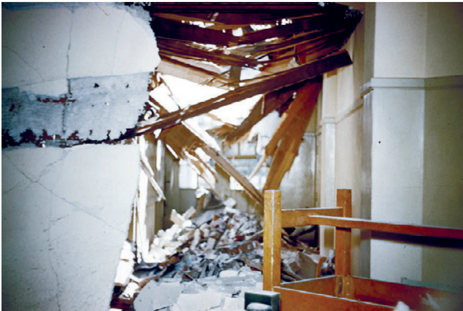
Figure 4-17: Destroyed exit corridor, Bakersfield, Kern County, CA, 1952
