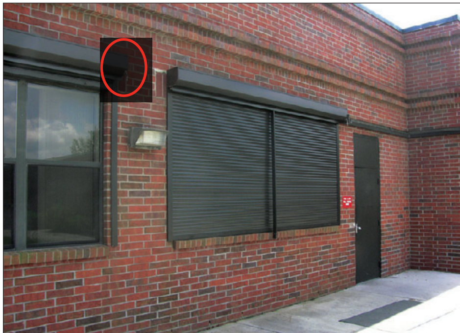
Figure 6-128: This school has roll-down shutters. The toggle in the red circle allows the shutter to be manually raised. Estimated wind speed: 130–140 mph. Hurricane Charley (Florida, 2004)
