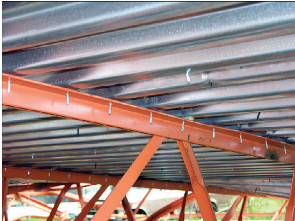
Figure 6-35: Even though the roof structure blew off, because of the strength and reliability of the screwed deck connections, the decking remained attached to the joists. Hurricane Charley (Florida, 2004)
