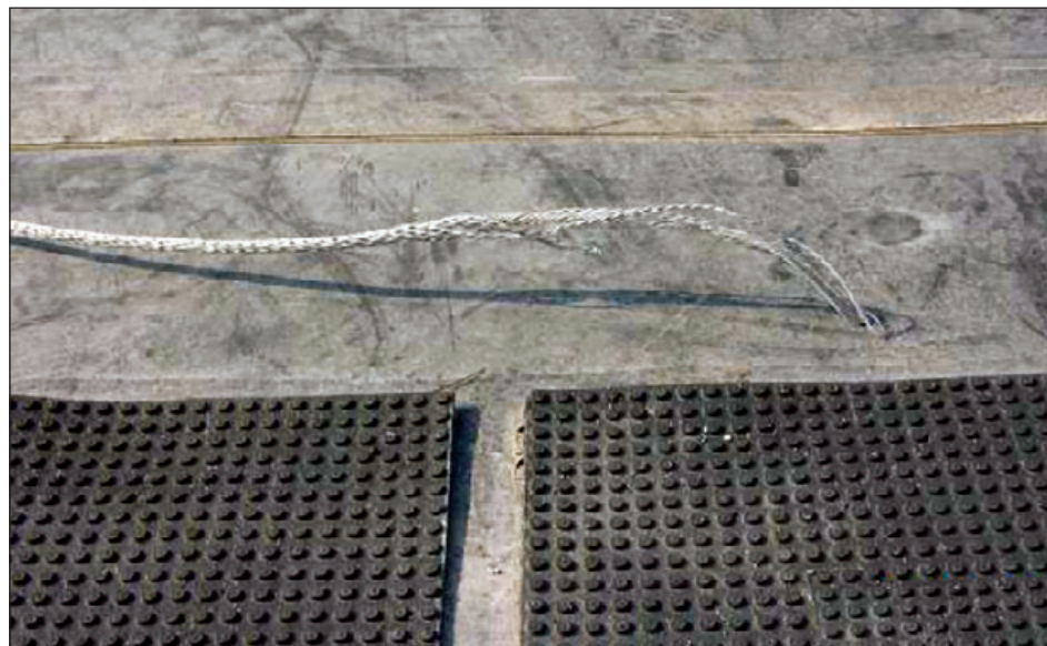
Figure 6-110: View of an end of a conductor that became disconnected. Estimated wind speed: 130 mph. Hurricane Katrina (Mississippi, 2005)
