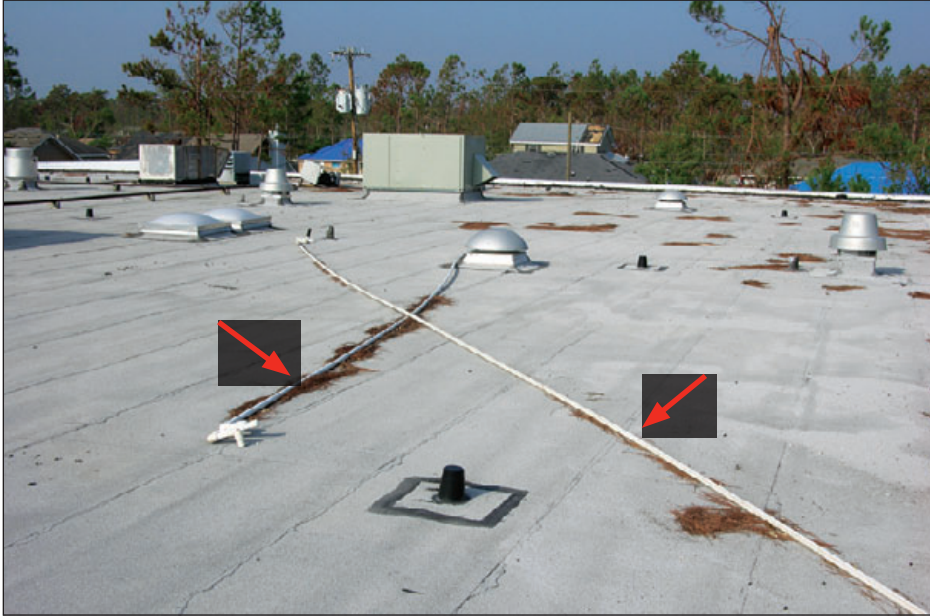
Figure 6-101: These two condensate drain lines detached from their HVAC units. They had not been anchored to the roof. Estimated wind speed: 125 mph. Hurricane Katrina (Mississippi, 2005)
