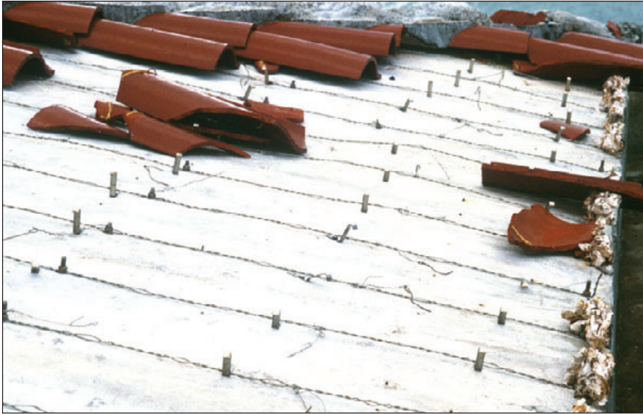
Figure 6-84 These wire-tied tiles were installed over a concrete deck. The failure was attributed to lack of vertical restraint, which allowed the tiles to lift and then be broken when they slammed back down onto the deck. Typhoon Paka (Guam, 1997)
