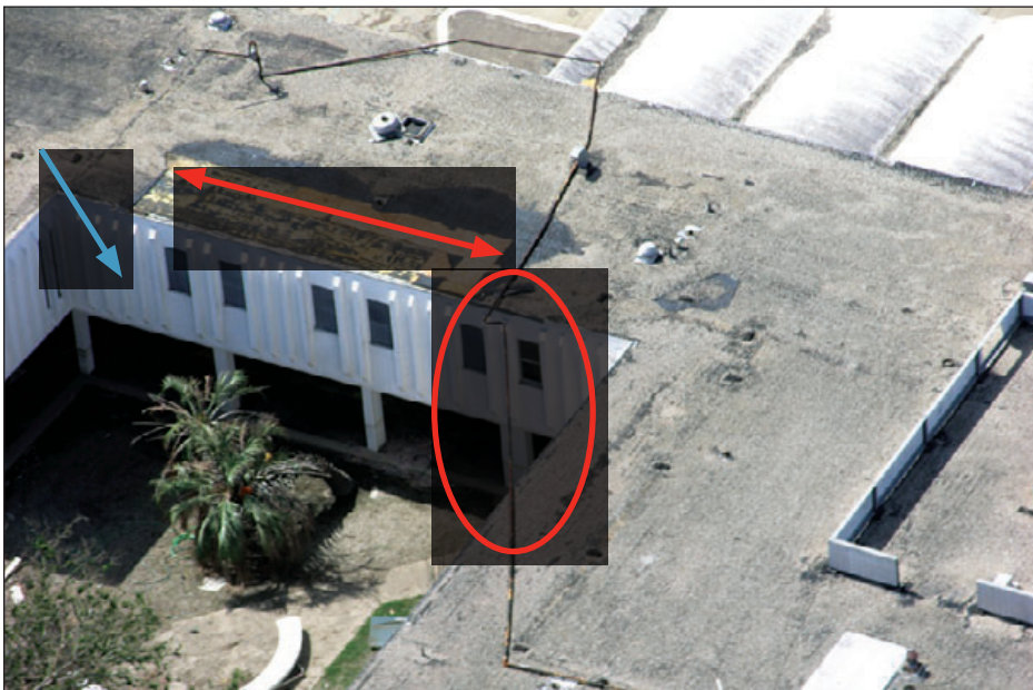
Figure 6-57: Although uncommon for schools, precast wall panels were attached to the structural frame of this school. This type of wall typically offers excellent wind performance. Note the roof covering damage and displaced gas line. Estimated wind speed: Approximately 125–130 mph. Hurricane Katrina (Louisiana, 2005)
