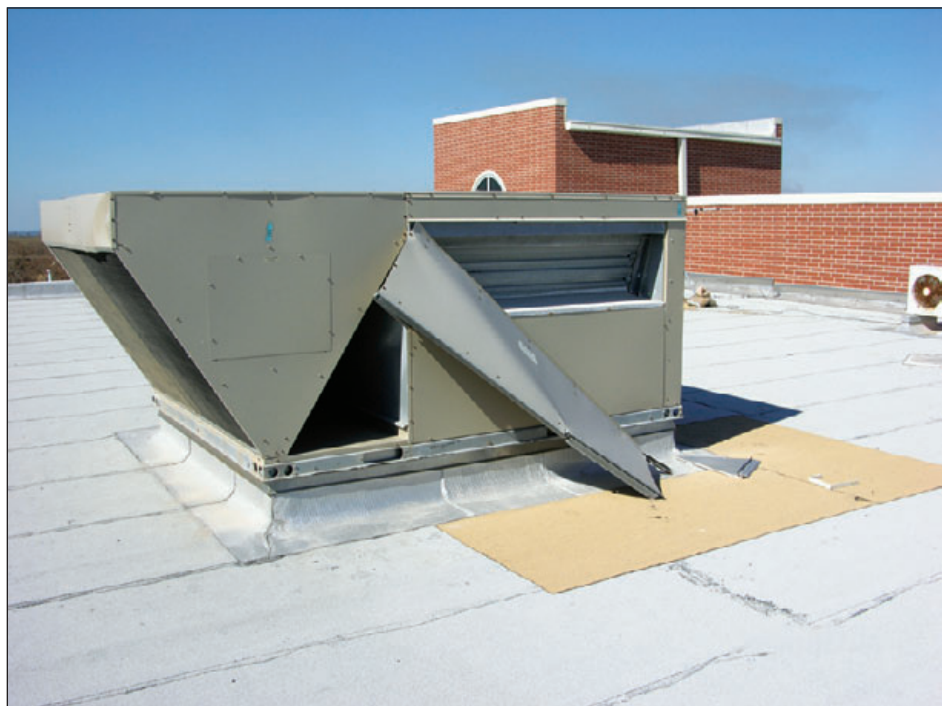
Figure 6-136: At this school, the hood on this HVAC unit was inadequately attached. A strap between the hood and unit can be economically installed to avoid this problem. Estimated wind speed: 110 mph. Hurricane Ike (Texas, 2008)
