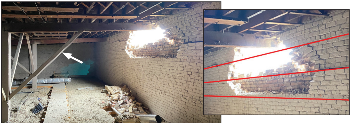
Damage to a URM building in downtown Salt Lake City from the 2020 Magna earthquake. The image shows unreinforced brick with header courses (red lines). The wall has out-of-plane masonry damage. The diagonal brace (white arrow) was strong enough to support the roof beam preventing collapse of the roof framing. Photo courtesy of Reaveley Engineers.
