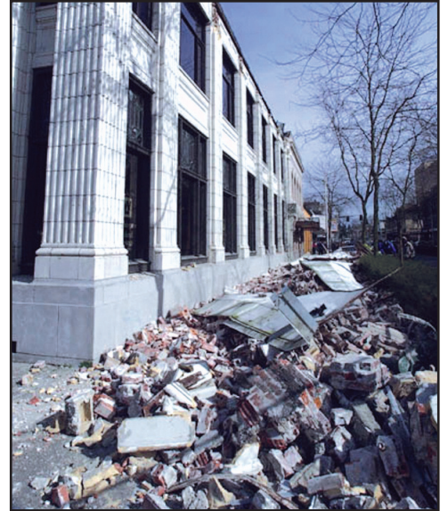
This bank was damaged in the Nisqually, Washington, earthquake, requiring customers to seek services elsewhere. Photo courtesy of The Olympian, Olympia, Washington.
