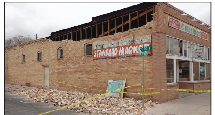
Structural damage to an unreinforced masonry building in downtown Magna caused by strong ground shaking from the Magna earthquake. Photo courtesy of the Utah Geological Survey.
