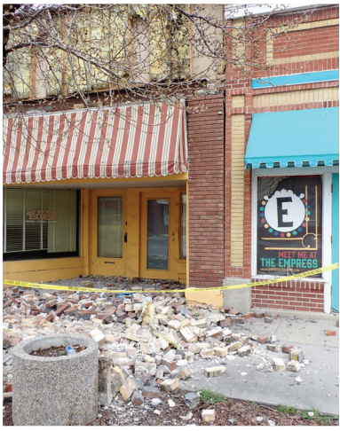
Damage in downtown Magna caused by the M 5.7 Magna earthquake of 2020. Photo courtesy of the Utah Geological Survey.
