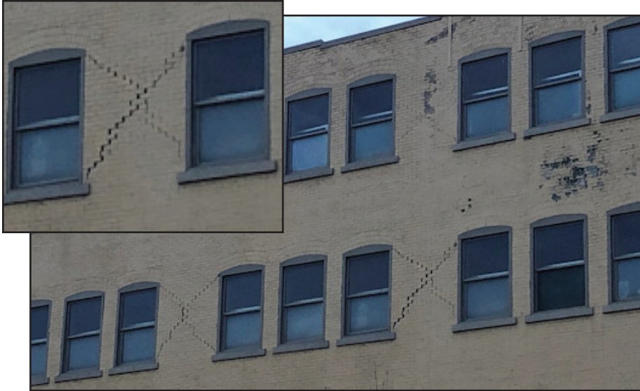
Damage to a URM building in downtown Salt Lake City from the 2020 Magna earthquake. The "X" pattern between the arched windows is a telltale sign of URM construction. This is an example of "in-plane" failure. Photo courtesy of Reaveley Engineers.
