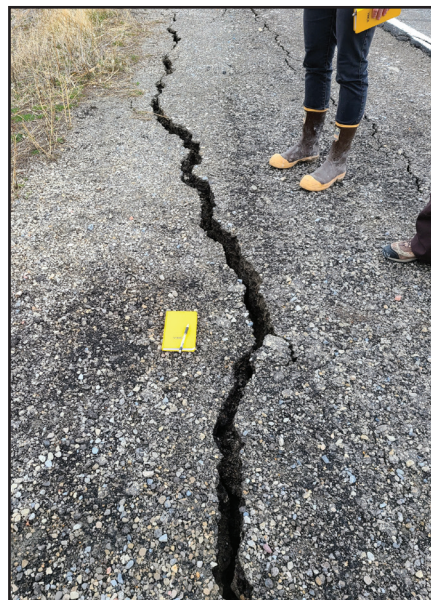
Lateral-spread ground cracking along the Great Salt Lake Marina access road from the Magna earthquake. Photo courtesy of the Utah Geological Survey.
