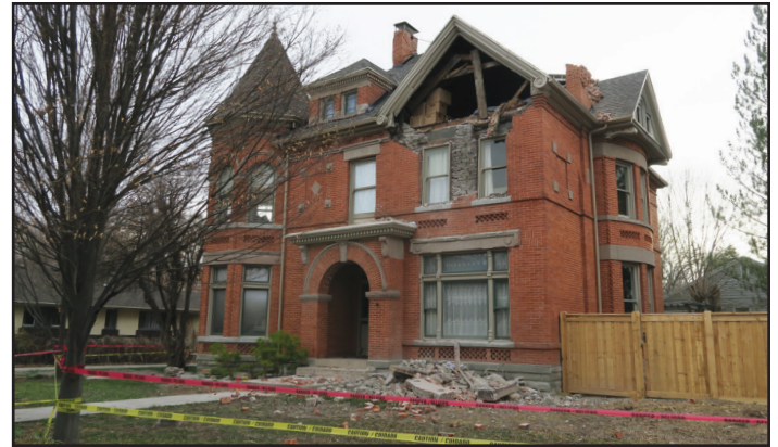
Structural damage from ground shaking to the historical Sears Mansion in Salt Lake City. This home was subsequently demolished due to the extensive damage. Photo courtesy of the Utah Geological Survey.
