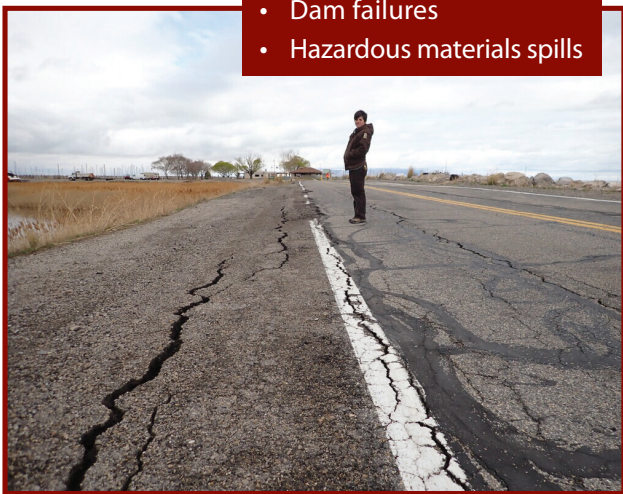
Cracks and road damage along the Great Salt Lake Marina access road likely from the 2020 M 5.7 Magna, Utah earthquake. Photo courtesy of the Utah Geological Survey.
