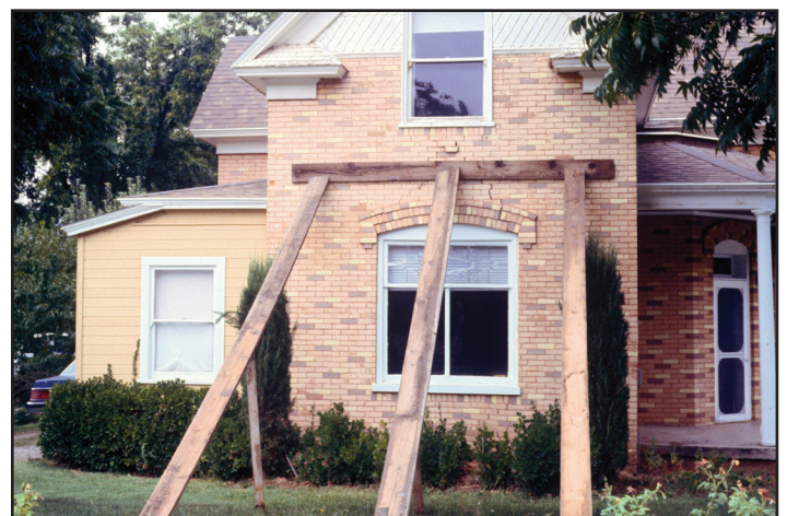
Bracing of an unreinforced masonry home damaged by the 1992 St. George earthquake. Cracks can be seen between the first and second story windows. Photo courtesy of the Utah Geological Survey.
