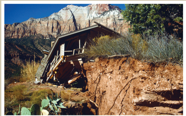
Home destroyed by the Springdale landslide, triggered by the September 2, 1992, M 5.5 St. George earthquake. Photo courtesy of the Utah Geological Survey.
